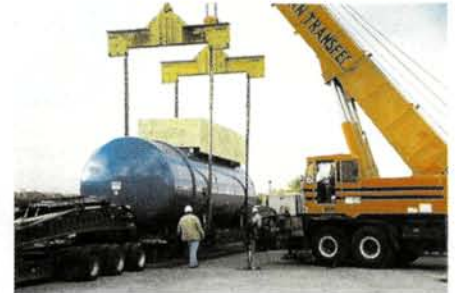
Coldbox ready to load on special low clearance trailer
